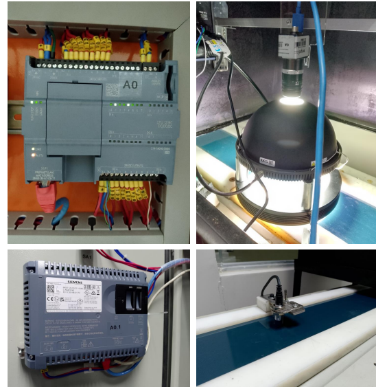
Figure 2: (top-left) Siemens S7 1200 PLC. (bottom-left) HMI TP700 comfort. (top-right) Vision system and lighting system. (bottom-right) Inductive Sensor.
