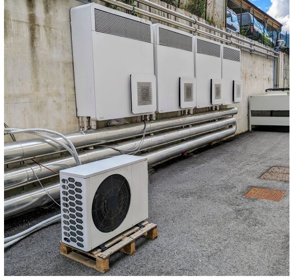
Figure 1: The water-air heat pump under test in the experimental field.
