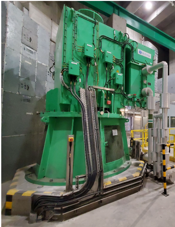
Figure 2: The motor that drives one of the pumps in main pumping station 2.
