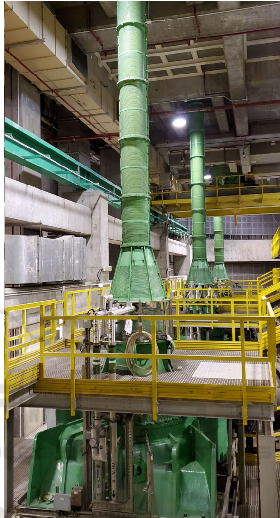
Figure 3: Main pump body that transfers sewage from the collection tunnels to the treatment pools 40 meters above.
