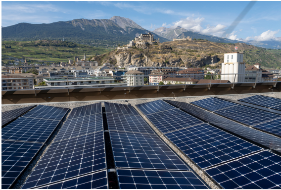
Figure 3: The studied system in Sion, Switzerland.
