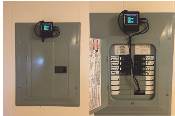
Figure 3: A SPM meter is installed in the circuit breaker box of a home taking part in the pilot project.
