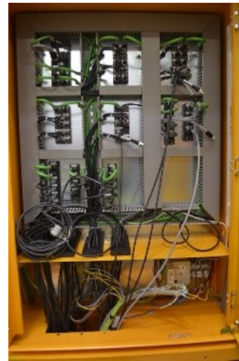
Figure 4: Distributed I/O Panel.
