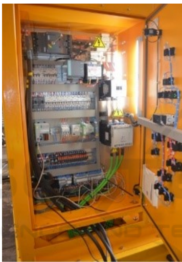
Figure 3: Power and Control Panel.
